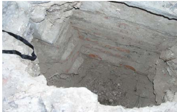
Figure 3 – Stone foundations have been adequate to support high loadings for hundreds of years
