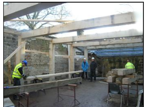
Figure 2 – A simple hardwood timber frame replacing steel saved 16 tonnes of CO 2 in this building.
